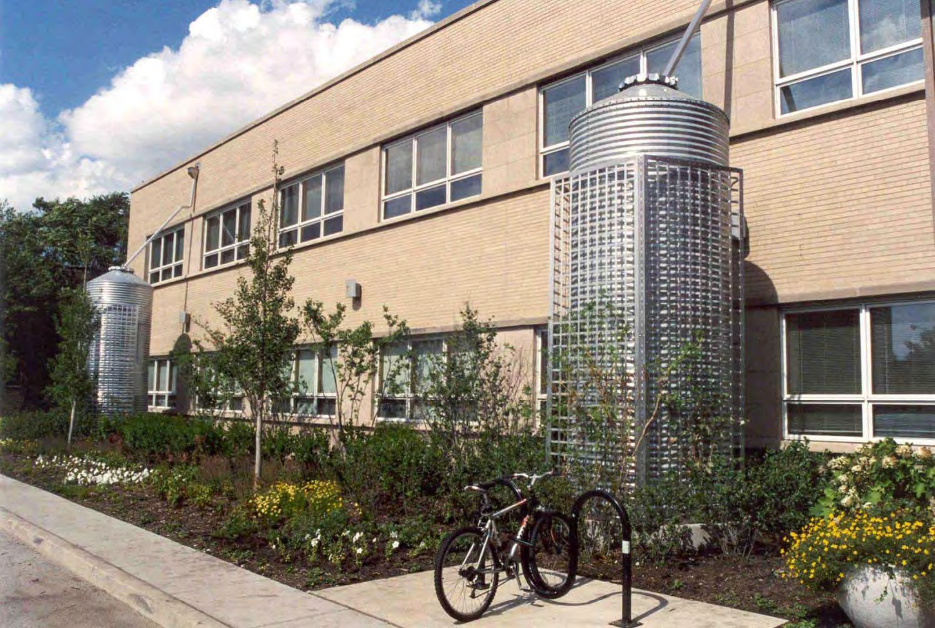
Downspouts, rain barrels, and cisterns
